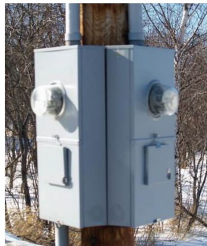
Minnesota Power overhead lot line meter base installation
