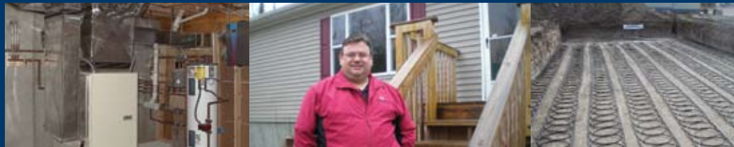
Left to right: a GSHP in a residential setting can meet 100% of heating and cooling needs; homeowner Jim Swanson is a true believer in GSHP after installing one at his rural Duluth home; a horizontal slinky loop field being installed.
