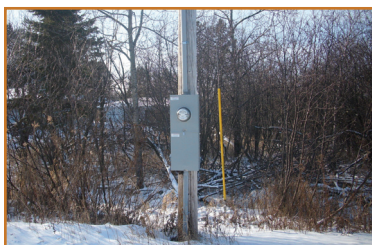
Meter enclosure on power pole
