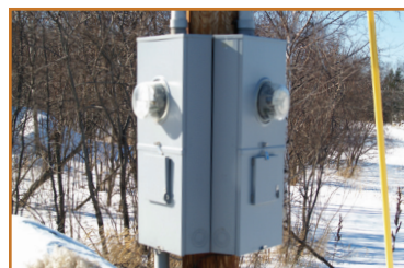
Meter enclosures on power pole
