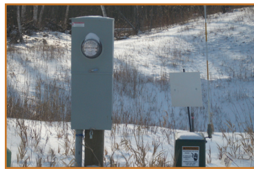
Secondary pedestal with meter pedestal
