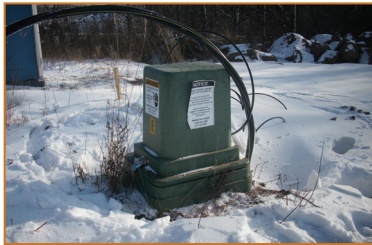
Secondary pedestal with conductors
