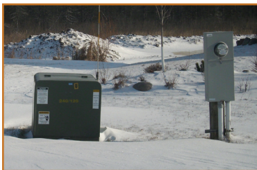
Pad-mounted transformer with lot line meter pedestal
